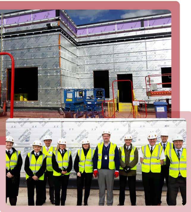
Visit to the new shared police and fire Operations Communications Centre, currently under construction at Hindlip
